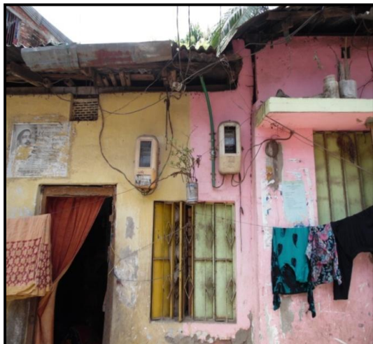
Figure 2.32: Electric meter is kept unprotected outside of the house, Chanmari bi lane, Motijhorna. Source: Field survey, August, 2014
