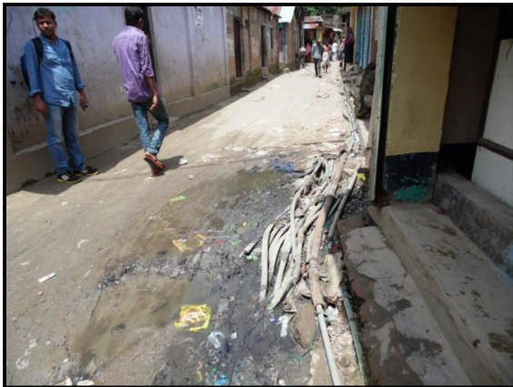
Figure 2.30: Poor management of water pipelines, Tankir pahar, Motijhorna area Source: Field survey, August, 2014
