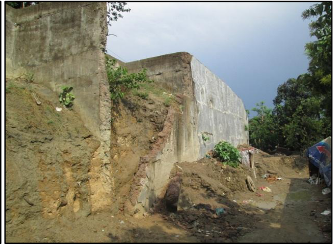
Figure 5.6. Retaining wall failure
