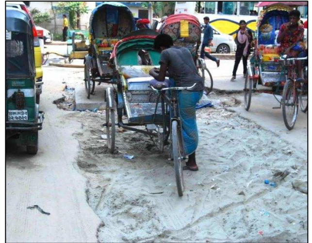
Photograph 8: Damaged Road Condition
