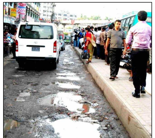
Photograph 24: Damaged Road Condition
