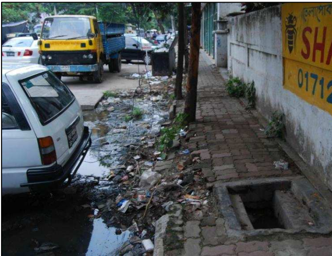
Photograph 3: Open Slab of Drain on Footpath
