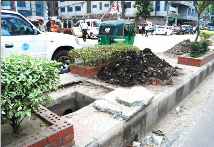
Photograph 7: Open Pit on Median Separation
