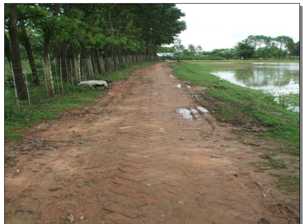
Photograph 06: Poor road way condition
