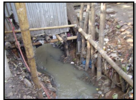
Photograph 4.11: Latrine above Drains
